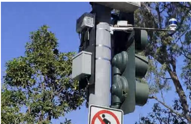
Fig. 3 Installation example: Lidar-IIS solution from Velodyne Lidar, powered by Bluecity
